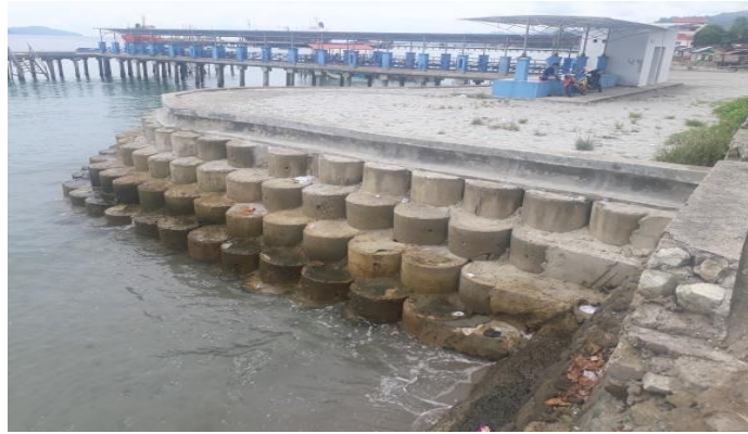
Figure 4. Construction of talud and jetty accelerated mangrove extinction (Photo: Manuel Kaya)
